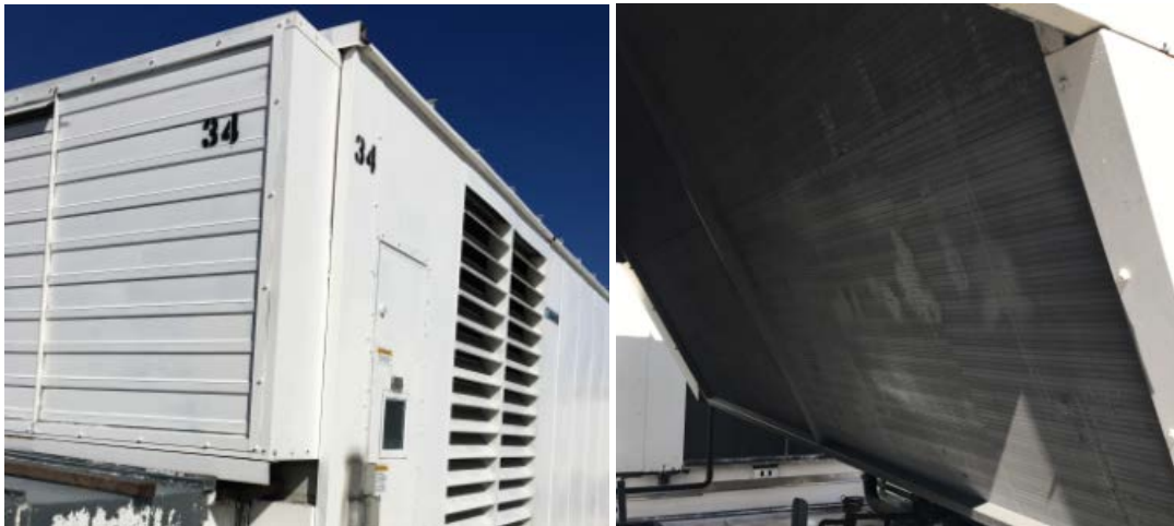
Figure 40 ACU-34, 170 tons, Condenser Face, Treated
