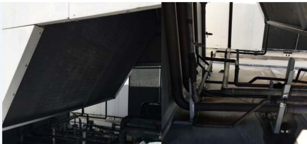
Figure 41 ACU-34 (cont'd), 170 tons, Condenser Face, Treated
