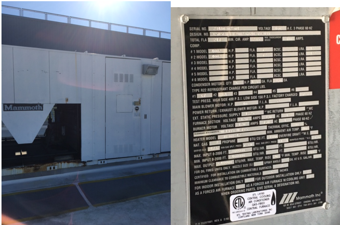
Figure 19 Mammoth ACU-11, 90 tons, Nameplate
