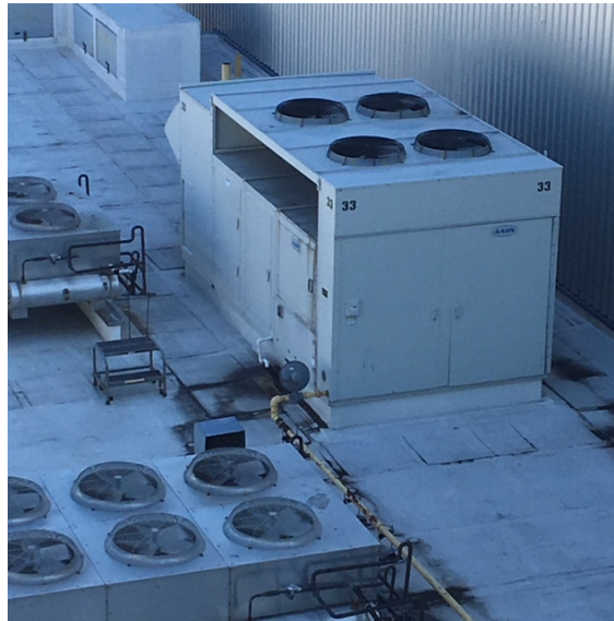
Figure 15 Aaon ACU-33, 40 tons
