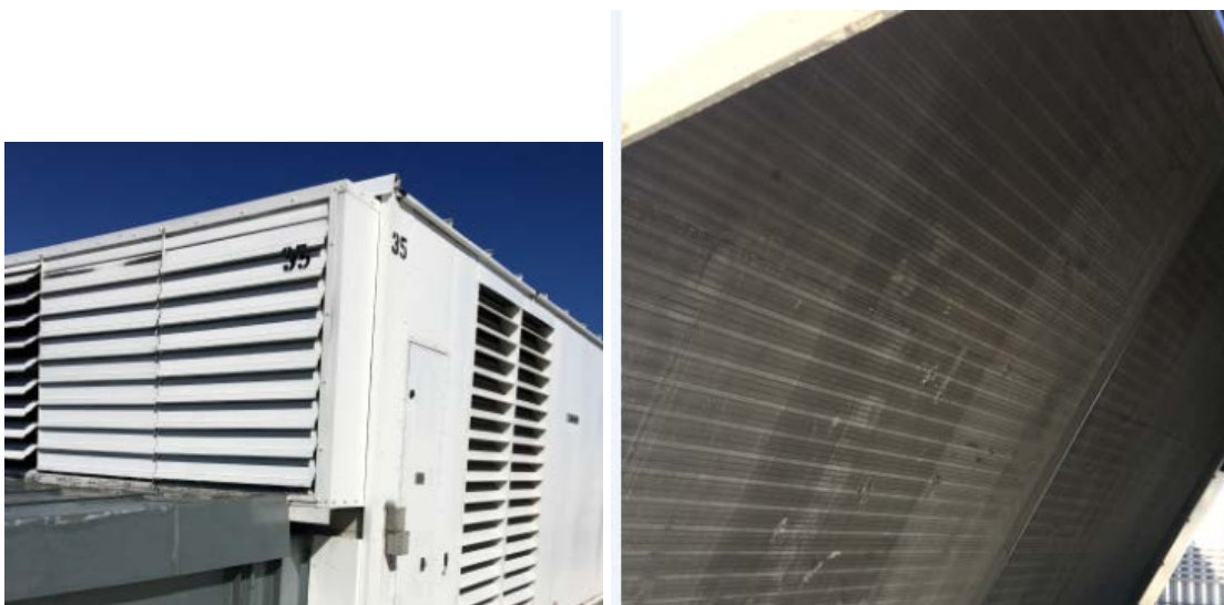
Figure 42 ACU-35, 170 tons, Condenser Face, Treated
