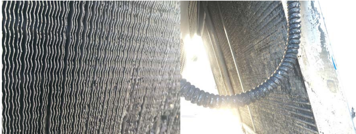
Figure 36 ACU-16, 40 tons, Condenser Face, Treated
