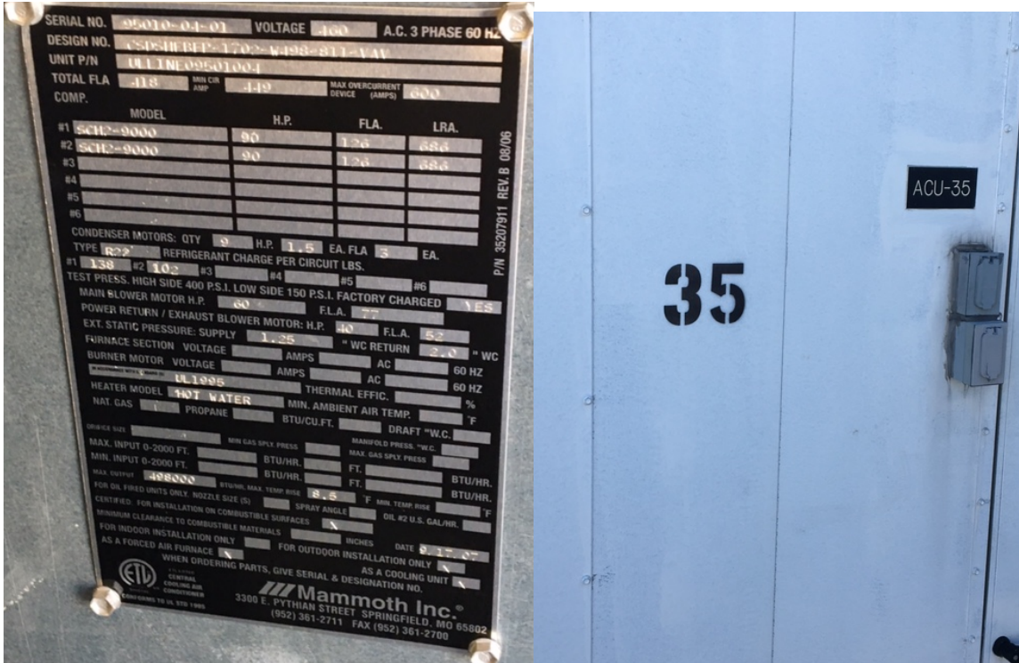
Figure 12 Mammoth ACU-35, 170 tons, Nameplate
