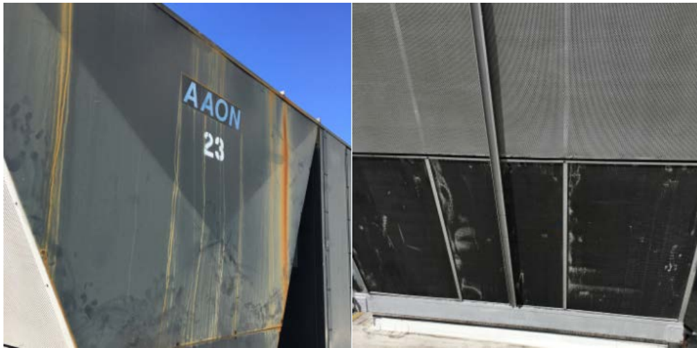
Figure 37 ACU-23, 50 tons, Condenser Face, Treated
