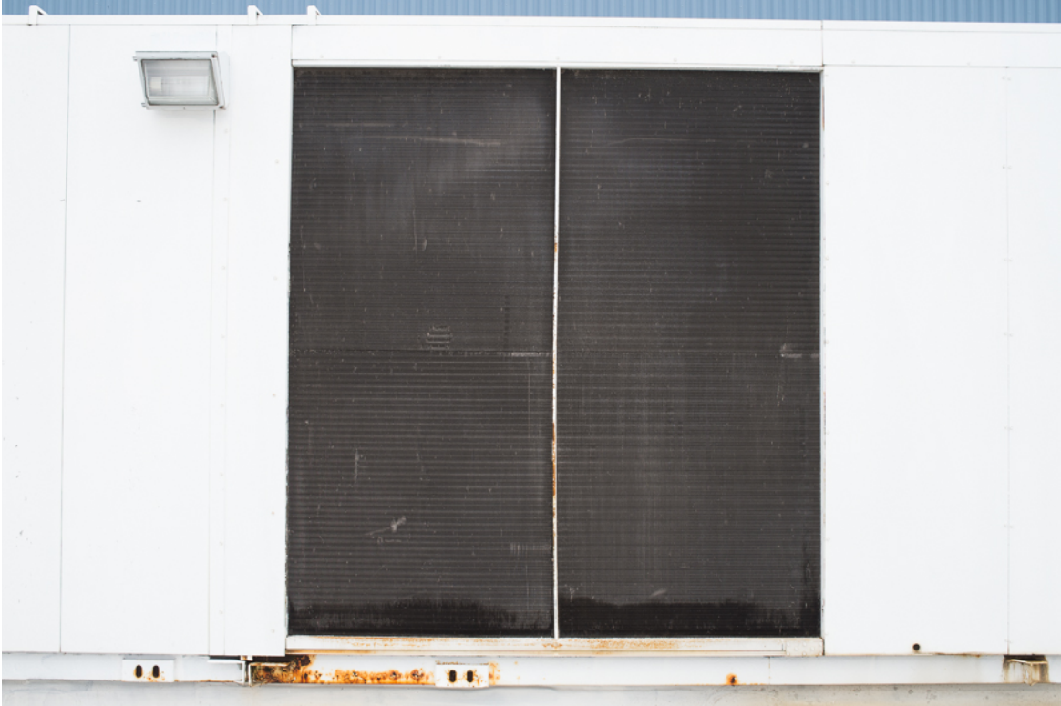
Figure 4 Mammoth ACU-14 Condenser Face, Untreated
