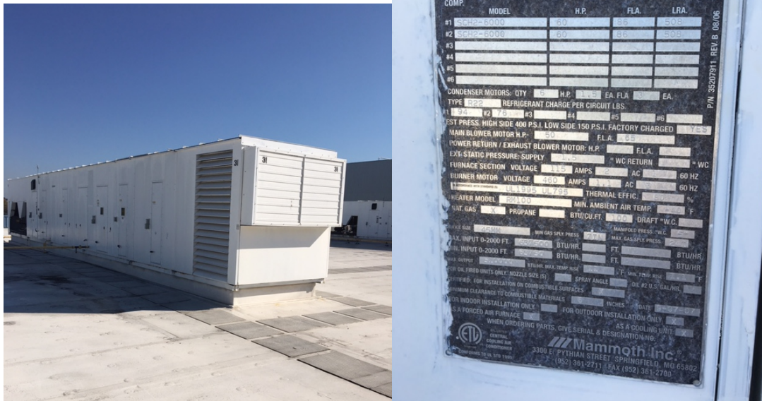
Figure 20 Mammoth ACU-31, 110 tons, Nameplate
