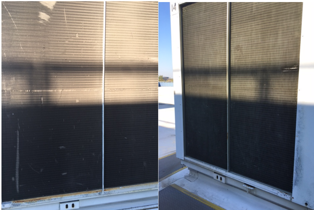
Figure 28 ACU-14, 160 tons, Condenser Face, Treated
