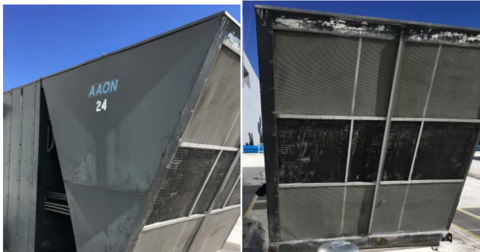
Figure 38 ACU-24, 70 tons, Condenser Face, Treated
