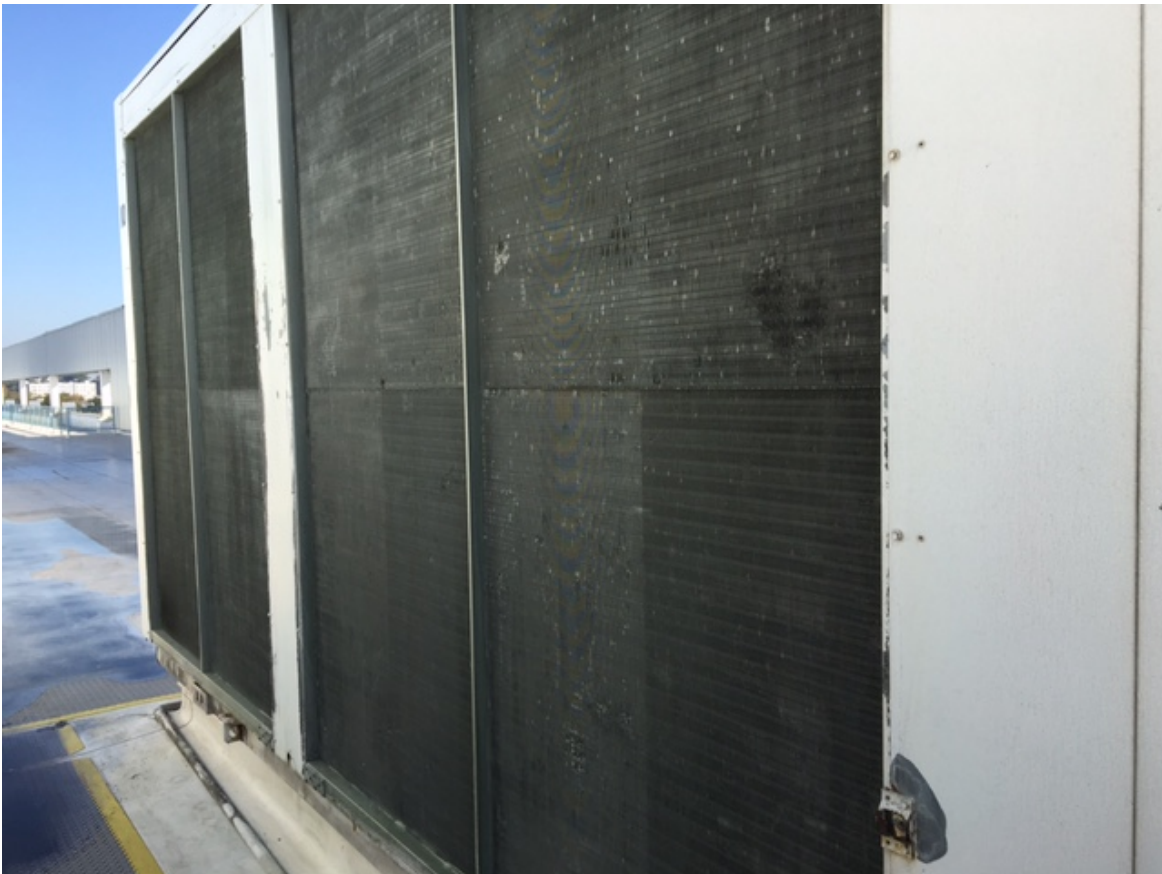
Figure 26 ACU-10, 150 tons, Condenser Face, Treated
