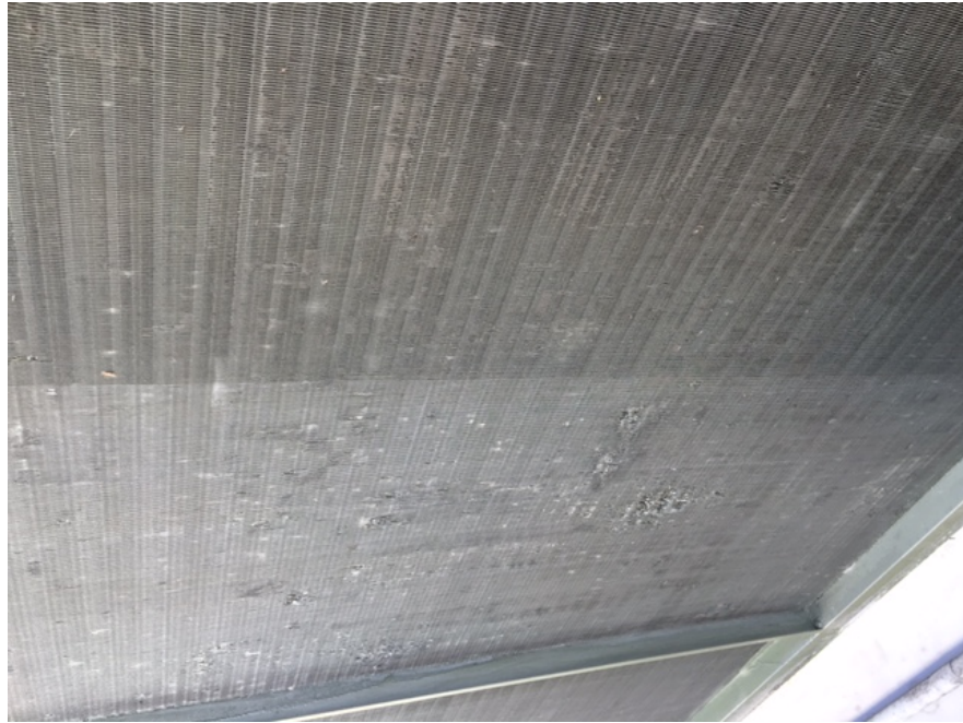
Figure 27 ACU-10, Condenser Face, Treated
