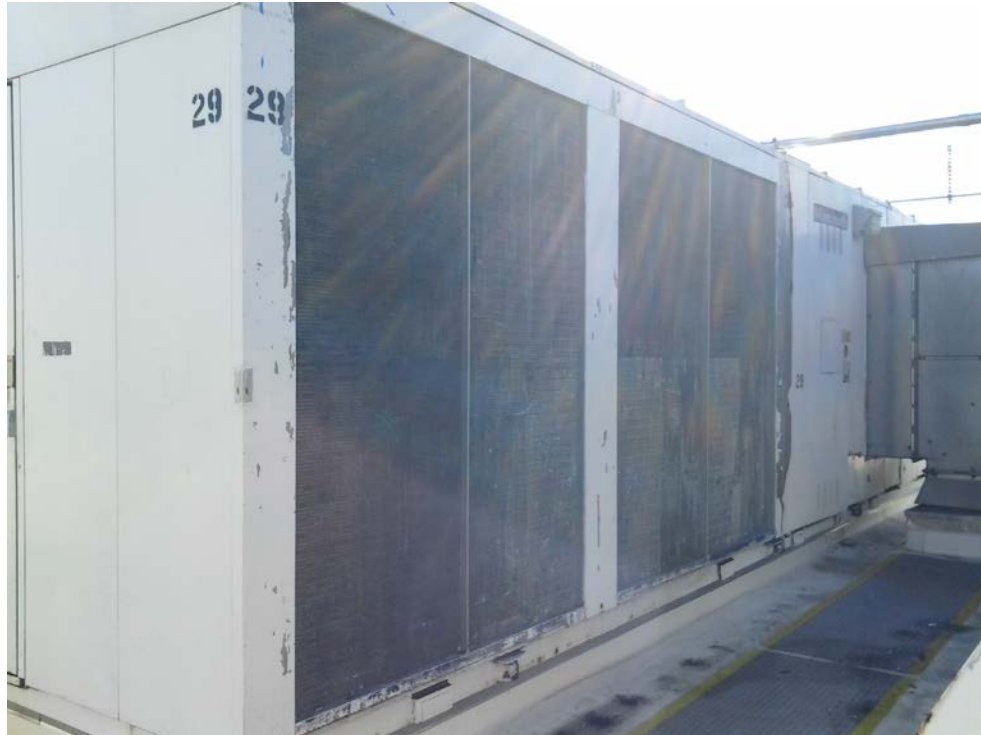
Figure 39 ACU-29, 150 tons, Condenser Face, Treated
