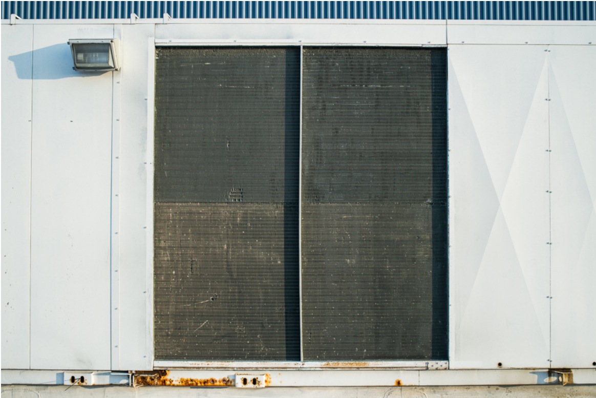
Figure 29 ACU-14, 160 tons, Condenser Face, Treated
