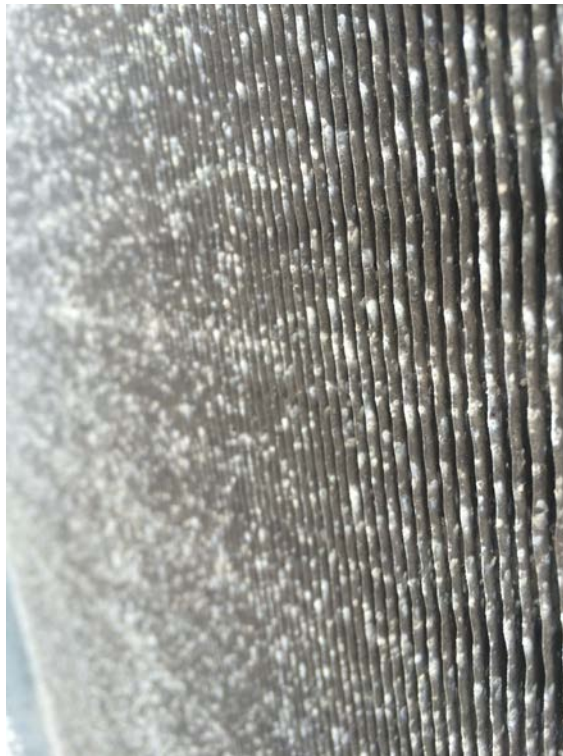
Figure 5 Mammoth ACU-14, Condenser Face, Untreated
