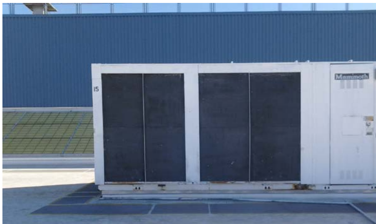
Figure 35 ACU-15, 160 tons, Condenser Face, Treated
